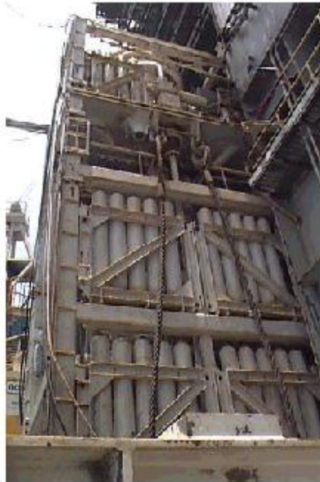
Subsea Accumulators Mounted on the BOP Stack
